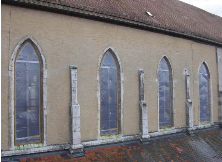
Fig. 2 - "Tape and Seal"-Technique: windows of a church are sealed with poly sheeting.
