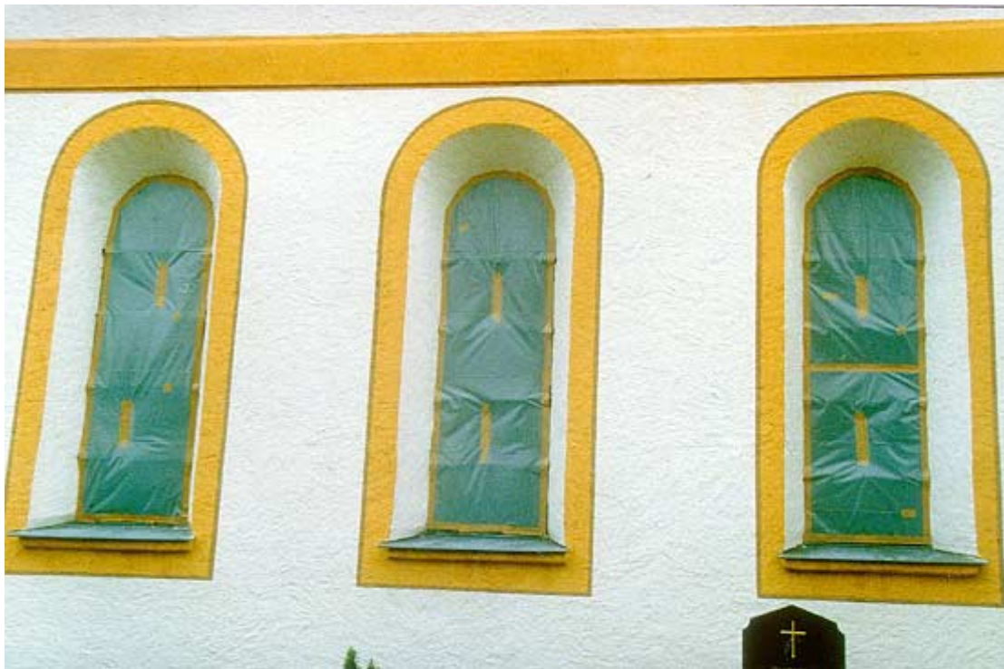
Fig. 3 "Tape and Seal"-Technique: windows of a church are sealed with poly sheeting
